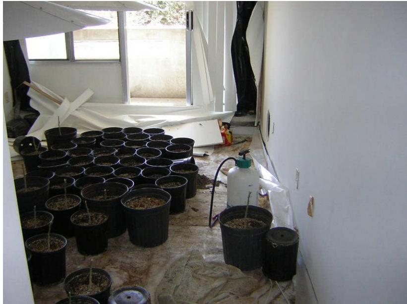
Illegal indoor marijuana cultivation, as in this grow-op discovered by police, can often produce serious levels of mould due to excess water leakage and moisture in the air
