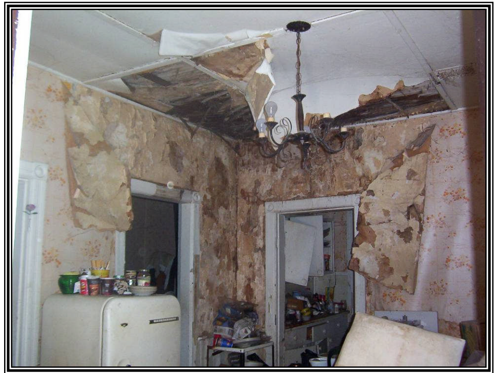
Mould infestation can cause enough damage to render a building uninhabitable.
